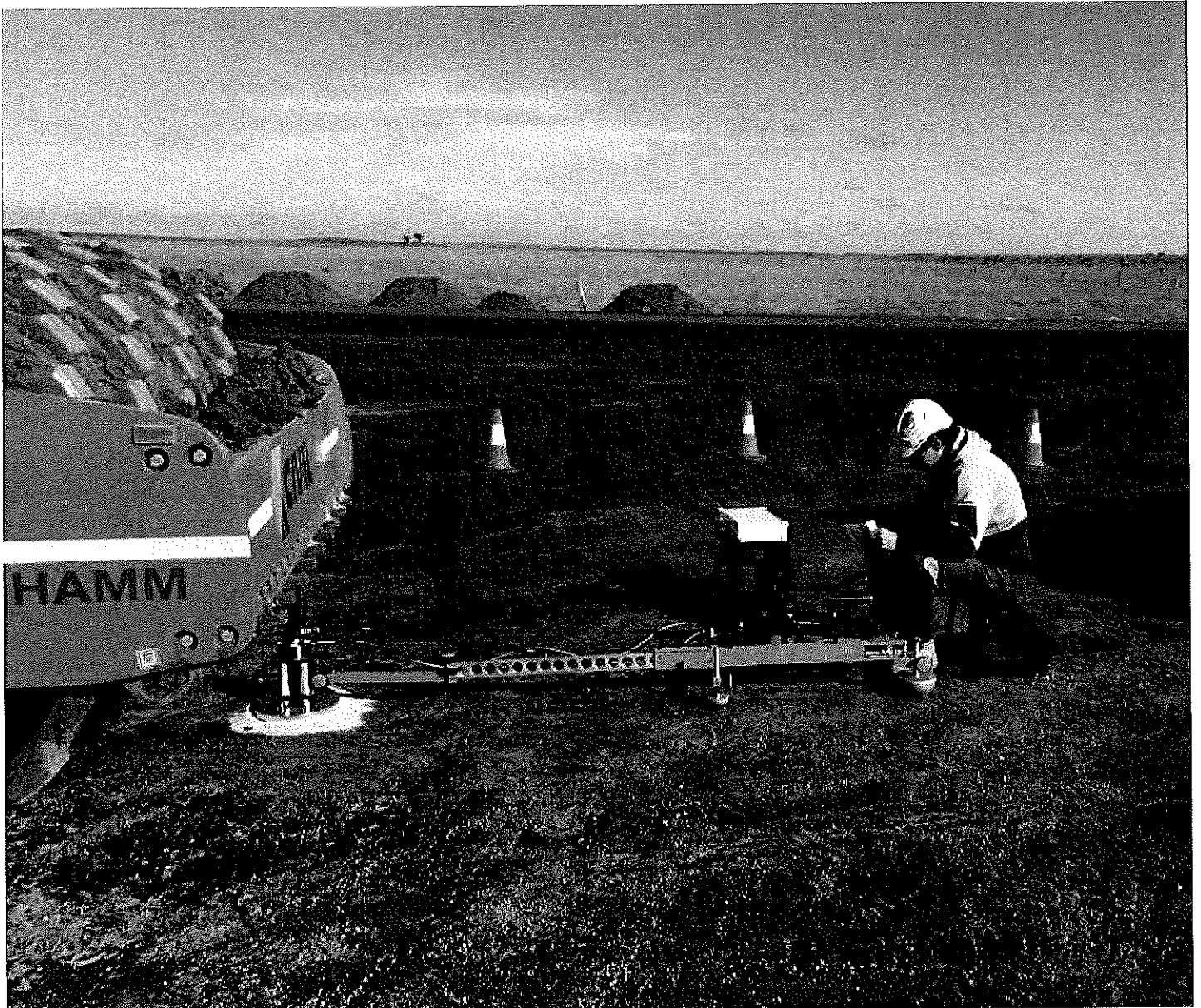
Plate Testing - to determine the allowable and ultimate bearing capacity of the ground.
