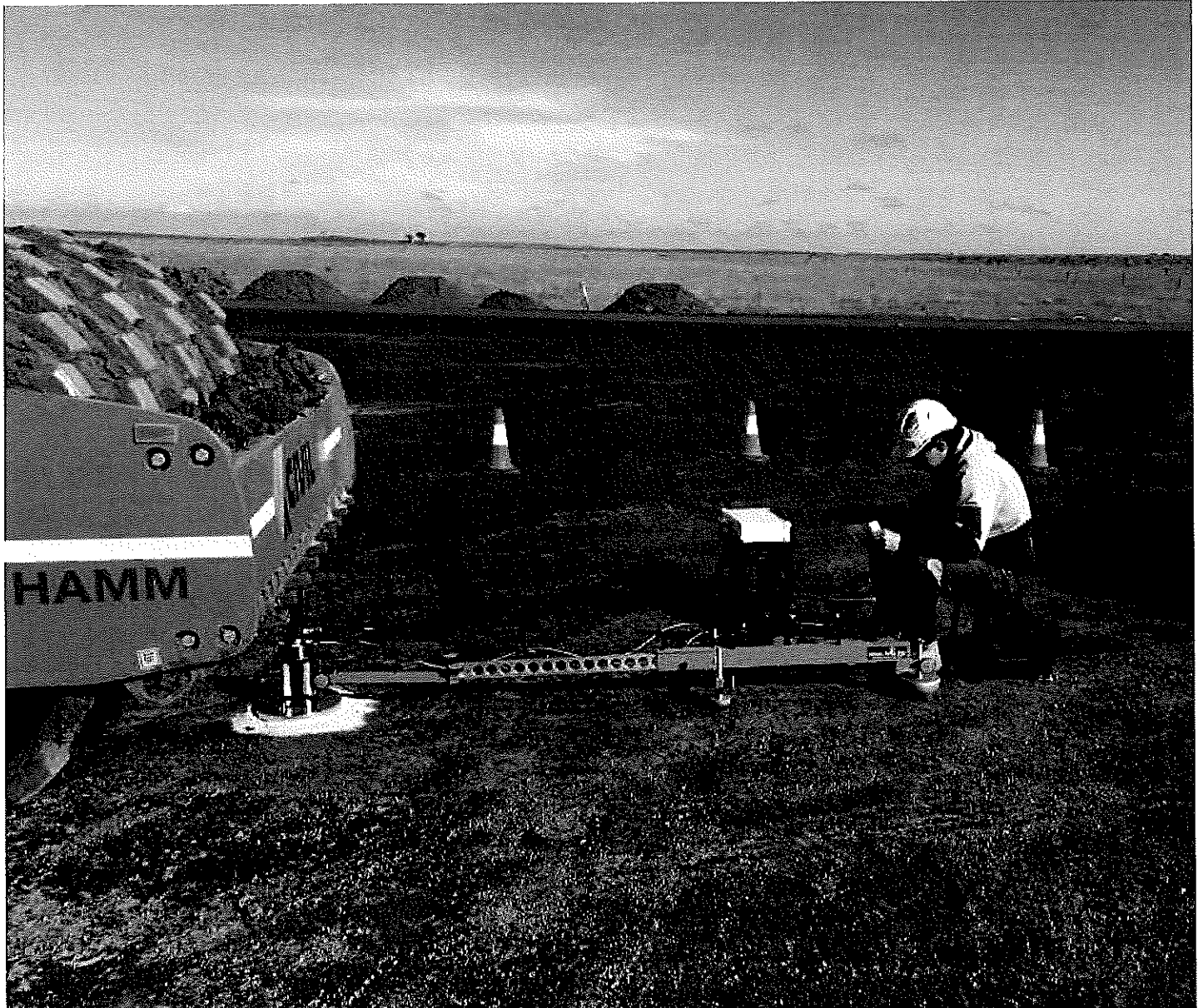
Plate Testing - to determine the allowable and ultimate bearing capacity of the ground.
